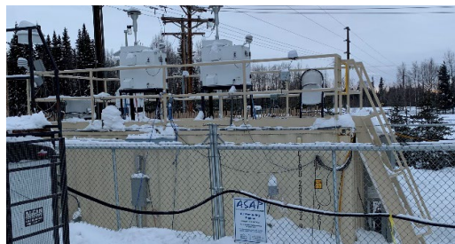
A particulate-matter monitoring station in Alaska. (EPA OIG photo)
